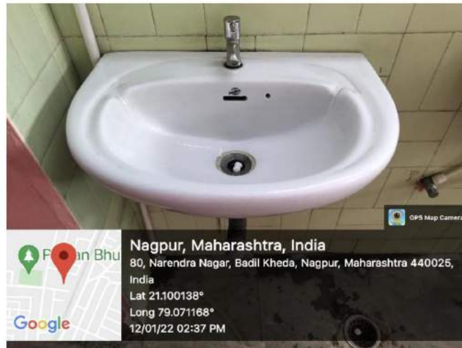
Taps to be replaced by Push Buttons
