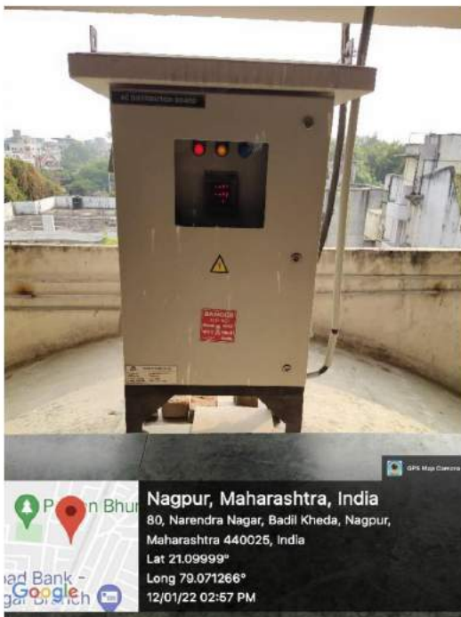
AC Distribution Board
