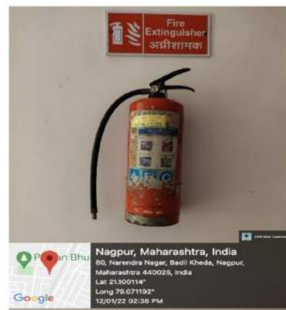
Fire Extinguishers in college
